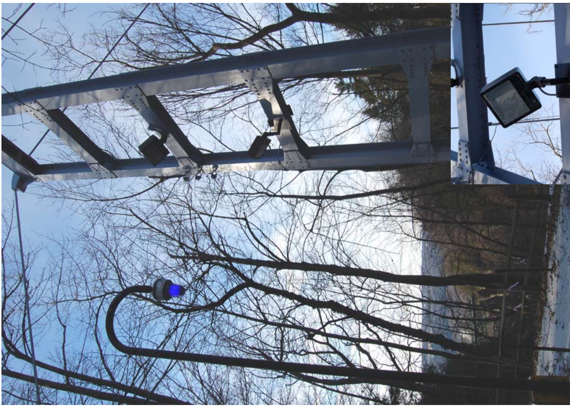
FLOOD LIGHTS MOUNTED TO SOUTH SUSPENSION BRIDGE TOWER
