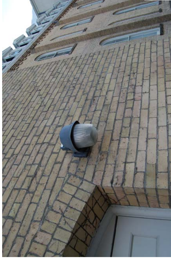
WALL MOUNTED FIXTURE ON NORTH FAÇADE OF SIBLEY HALL
