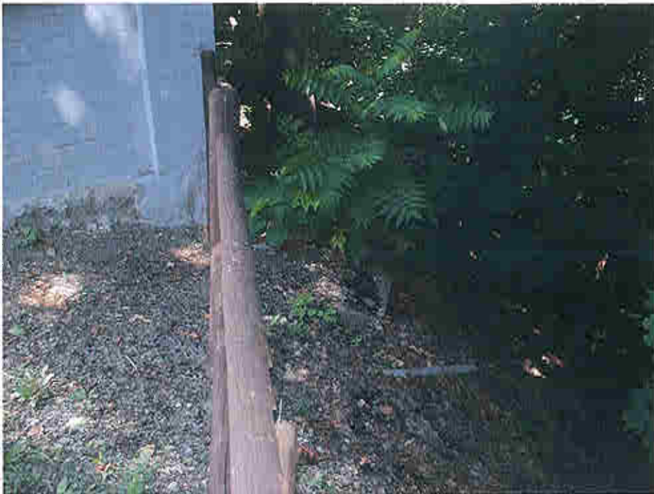
Photo 1 - Area where fresh concrete has been poured on grade surface in attempt to stabilize surface at NE corner Foundry.
