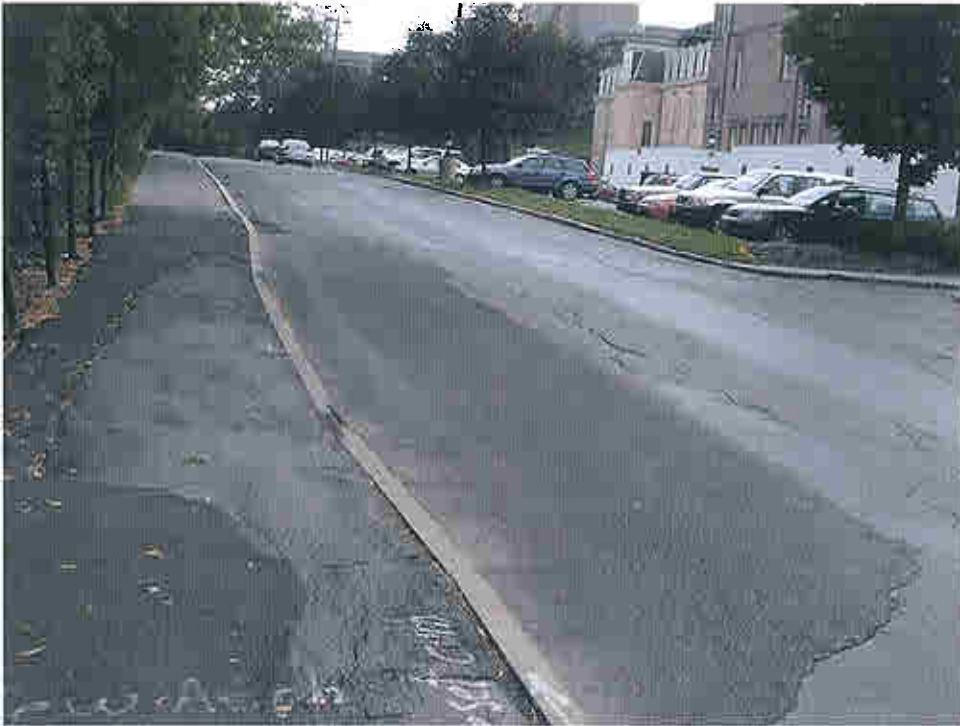
Photo 11 - Notice all of the pavement cracking along the North Curb line of University Avenue.
