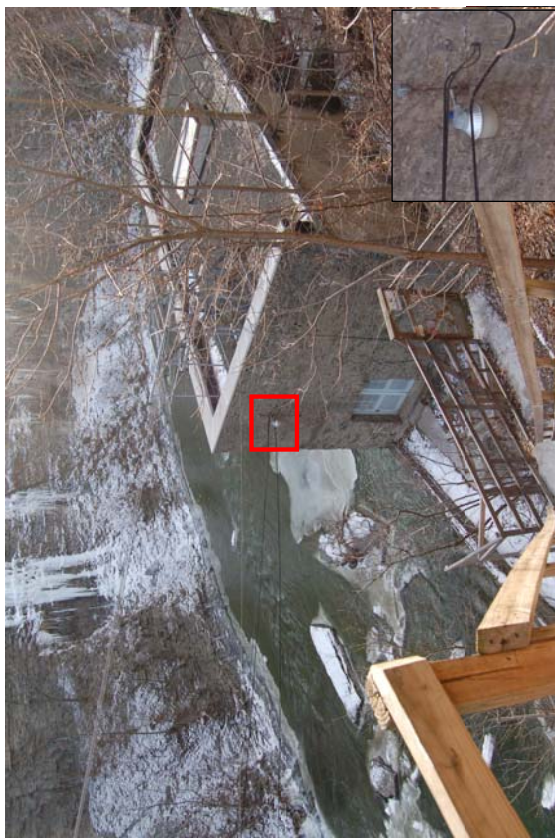
WALL MOUNTED FIXTURE ON HYDRO-ELECTRIC PLANT
