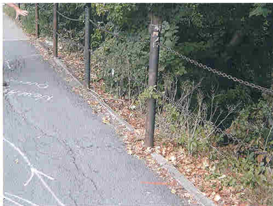
Photo 8 - This asphalt sidewalk has settled and the pavement appears to be translating northerly into the gorge
