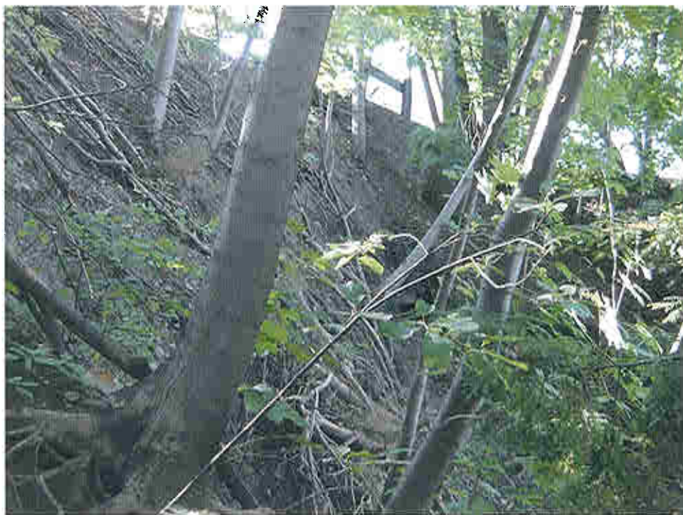
Photo 4 - Near vertical (and undercut barren earth face in danger of failure at any time. Foundry above left. Drain in Center.
