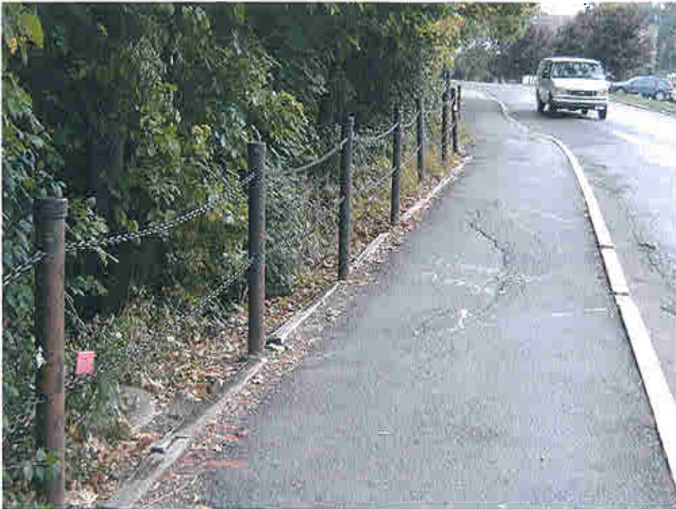
Photo 9 - A poor stormwater management practice and local slope failure area.
