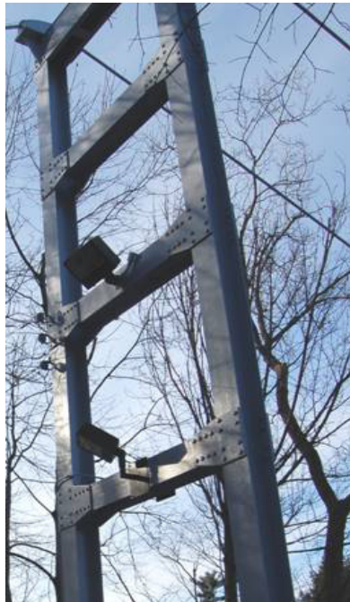
Figure 2.11.13: Suspension bridge flood lights.
