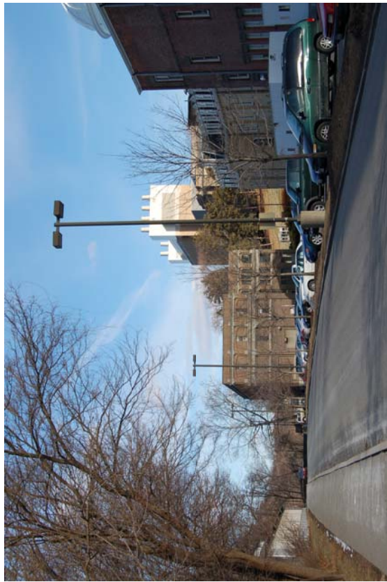
DUAL FIXTURE HEAD ON 30' POLE AT UNIVERSITY AVE
