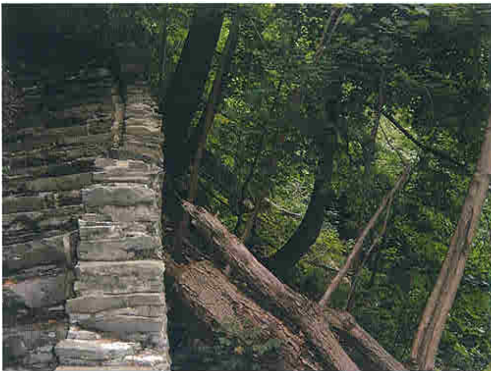
Photo 17 - Wet laid stone stair case on trail. Note rotation of wall to right and mortar in fill in gap between stairs and wall.
