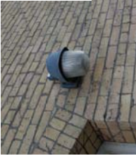
BUILDING MOUNTED LIGHT
