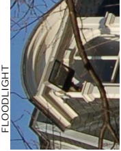
BUILDING MOUNTED FLOODLIGHT
