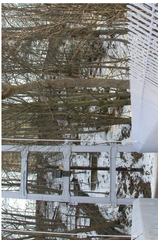
FLOOD LIGHTS MOUNTED TO SOUTH SUSPENSION BRIDGE TOWER
