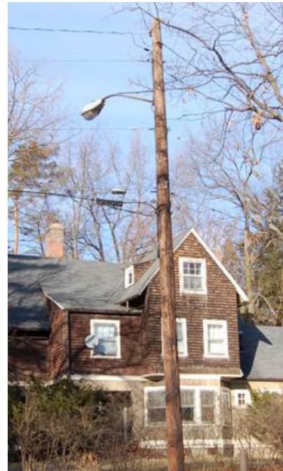
Figure 2.11.14: Cobra head street lights.
