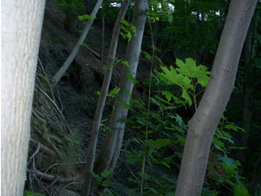
Slope NW of Foundry – note Drain Tile and undercut area at 10 o'clock. 07.13.07
