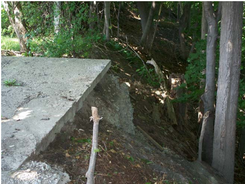
North edge of slab NW of Foundry – note concrete fill at center of photo. 07.13.07
