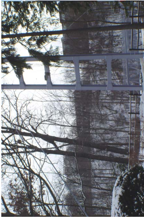
FLOOD LIGHT MOUNTED TO NORTH SUSPENSION BRIDGE TOWER
