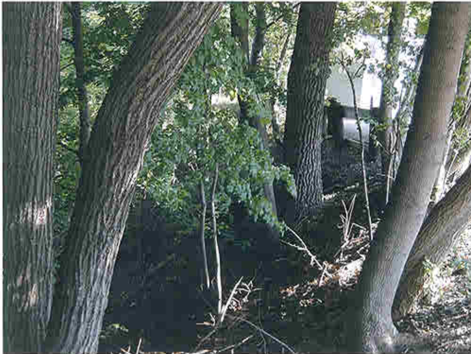
Photo 6 - Timber (poles) piles driven to retain slope, exhibit rotation northerly.
