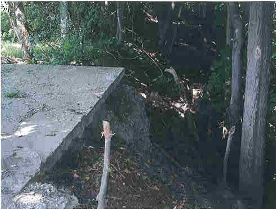
Photo 5 - Large mass of concrete fill exposed at NW corner of concrete pad. Note concrete poured on grade below (lower right).
