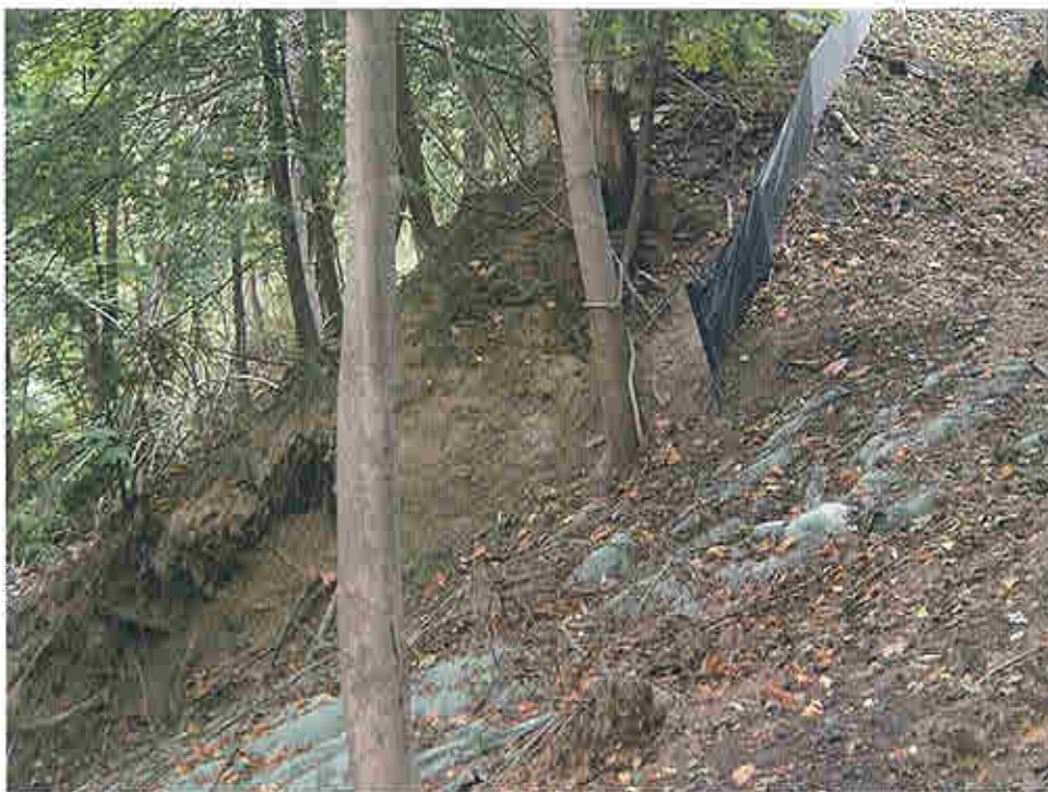
Photo 13 - Area of recently repaired local failure covered with erosion control fabric, but no planting of any kind are apparent.
