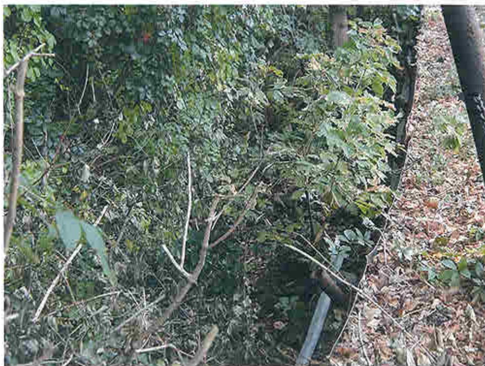
Photo 24 - Retaining structure at local slope failure area at University Avenue.
