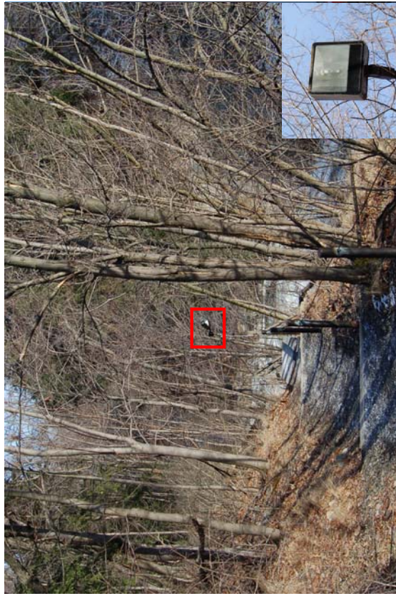
FLOOD LIGHT AT PATH TO HYDRO-ELECTRIC PLANT
