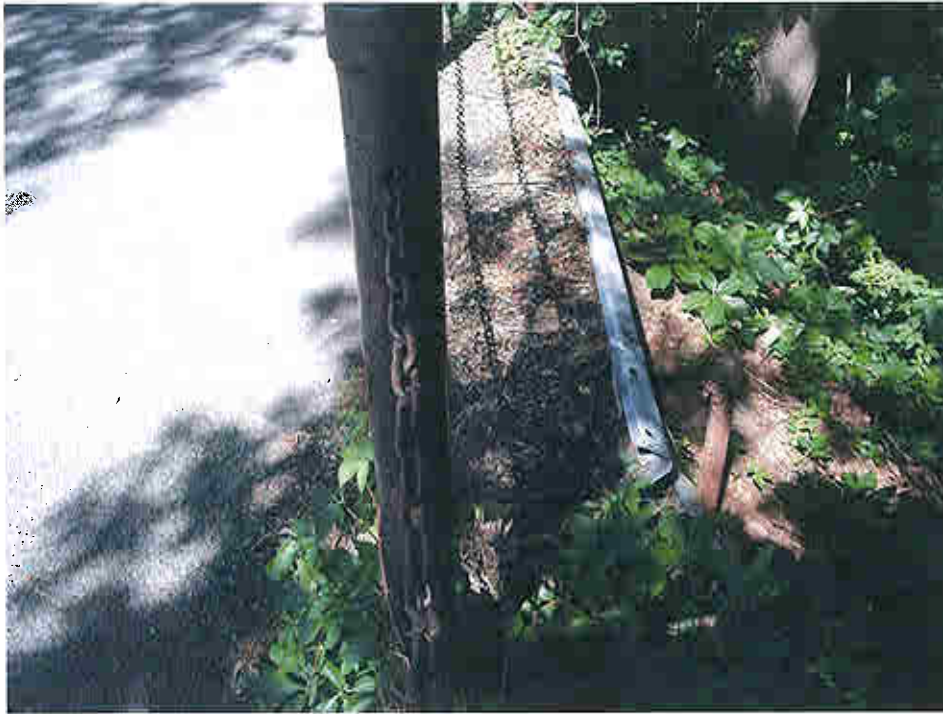
Photo 25 - Retaining structure at local slope failure area at University Avenue.
