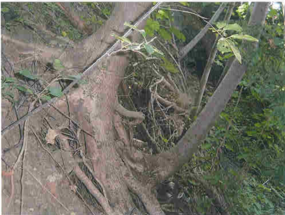
Photo 3 - Drain tile exposed at failed slope area.
