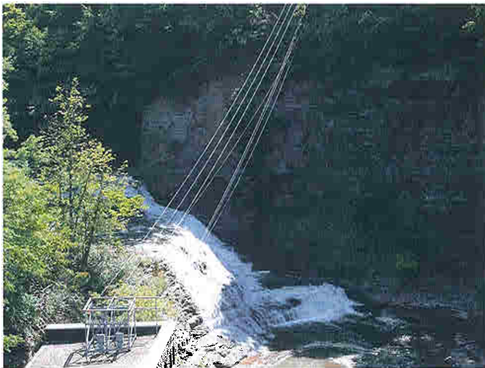
Photo 23 - Large rockface failure near edge of Falls.
