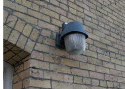
Figure 2.11.10: Building mounted light fixture/wall pack.
